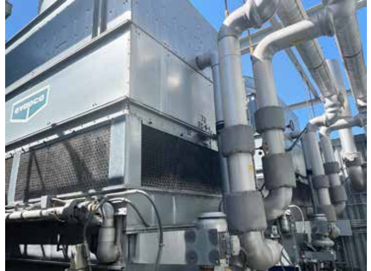
Cooling Towers on the roof – photo, M. Cullen
