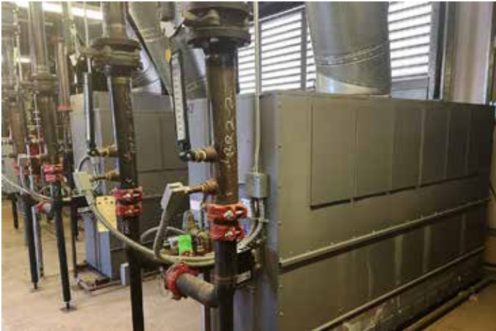
Rooftop boilers – photo, M. Cullen
