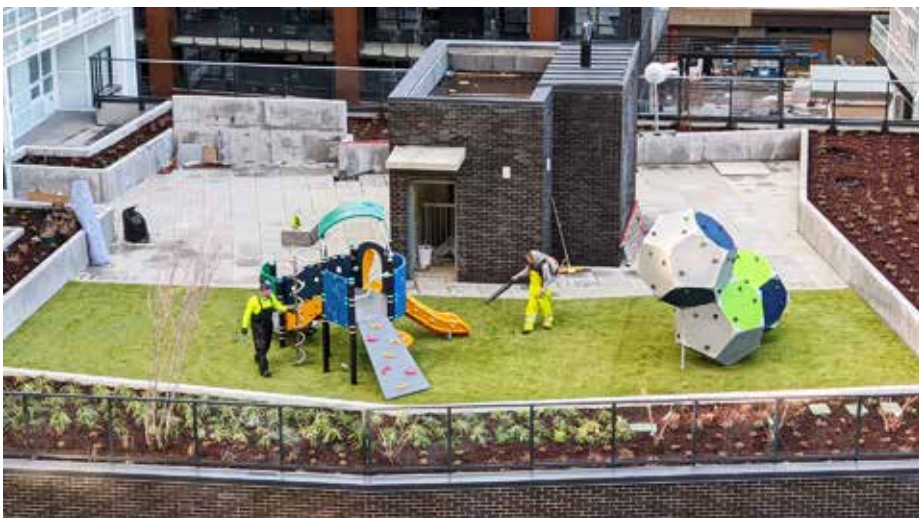
Workers in Onni's Fairview Avenue rooftop playground putting finishing touches on Astro Turf – photo, Julie Holland
