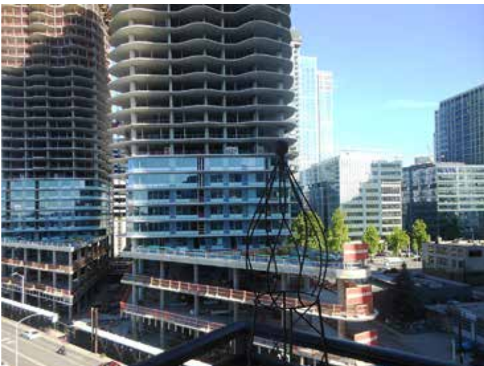
Westbank's towers southeast of Mirabella, and completed towers behind them – photo, M. Rogers
