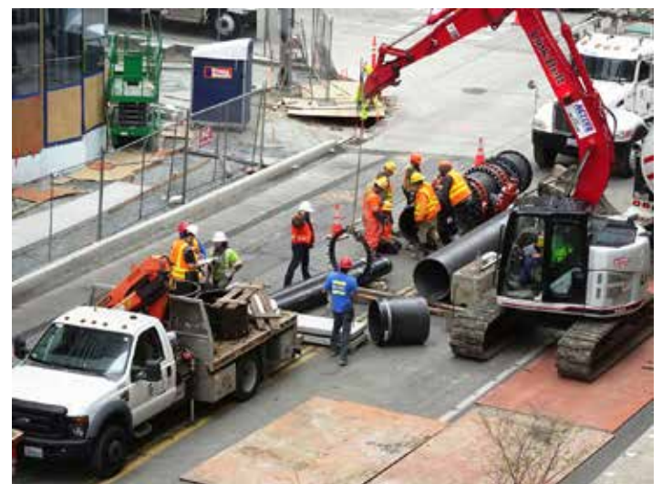
Following Seattle Public Utilities’ water main installation on Denny Way – L. Klein
