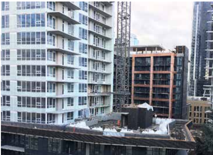
Onni South Tower deck holds bags of pavers ready to be installed – photo, J. Curtis
